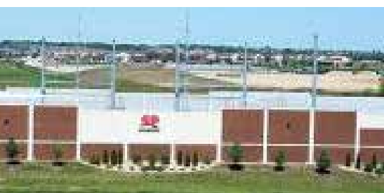
Utilities (SPU Substation)
